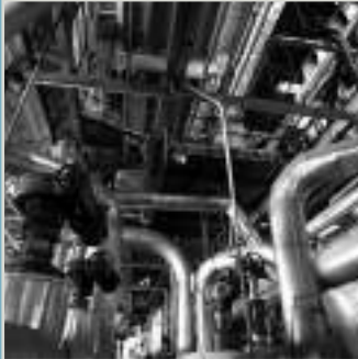
Pipeline for refrigerations or cooled media.
